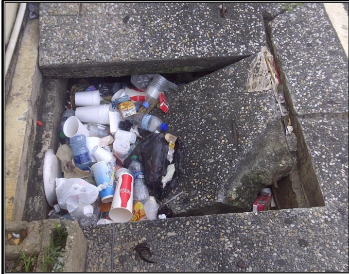
Litter accumulated within a broken pavement located in the borough of Arima causing a public nuisance to pedestrians.
